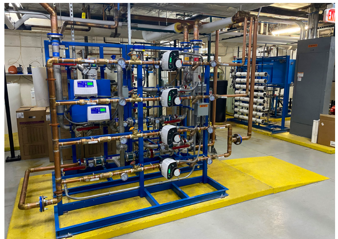
The MetroMix electronic mixing valve package arrived with the piping and valves factory mounted and wired. The duplex skid is accessible to the operation crew following a redesign of the piping installation.
