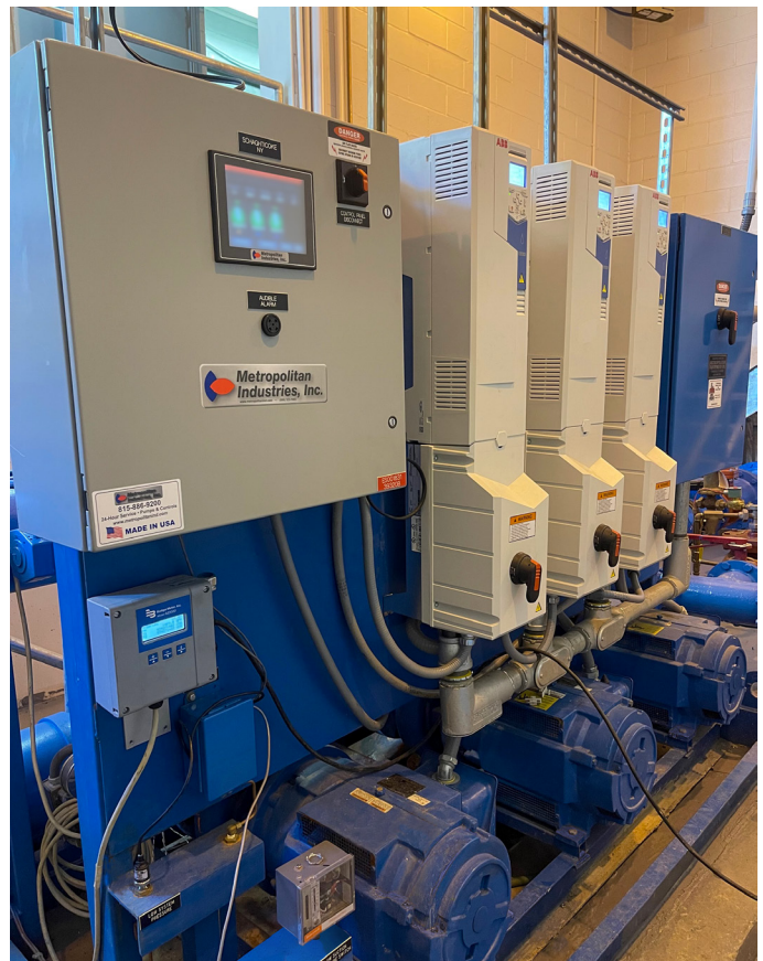
Newly installed control panel and VFDs customized to fit with existing equipment.
