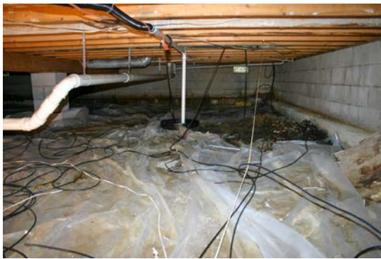
The removal of loose wires and excess debris across the crawl space floor is one of the several measures that should be addressed prior to encapsulating a crawl space.
