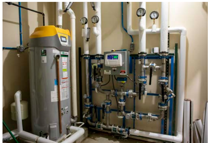
Right: MetroMix installation for a healthcare center in Champaign, Illinois.
