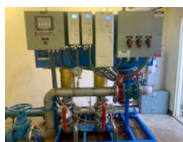
Booster Pump Skid Upgrade Improves Domestic & High Flow Capabilities to Upstate New York's 'Glove Cities' Pages 4
