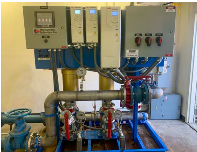
Booster system skid installed at Wesskum Woods.
