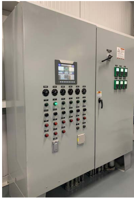
Left: Team leader Kim Emmons next to one of the newly installed pumps. Right: New 6 Pump Variable Speed Control Panel with double door enclosure.
