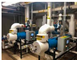
Preventative Solutions for Health Care Facility Remedy Unreliable Hot Water System Page 6
